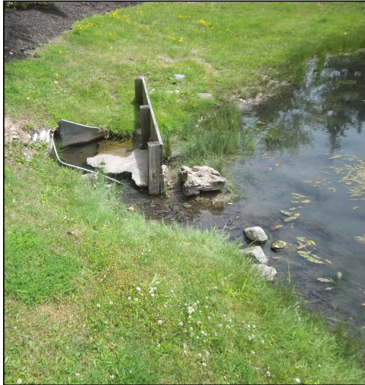
Figure 7. Existing pond's outlet structure lacks features that promote pollution removal.
