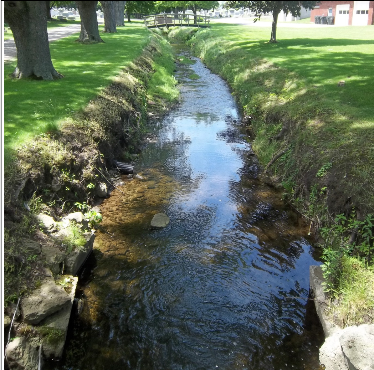
Figure 4. Eroded Streambank on Mill Creek.
