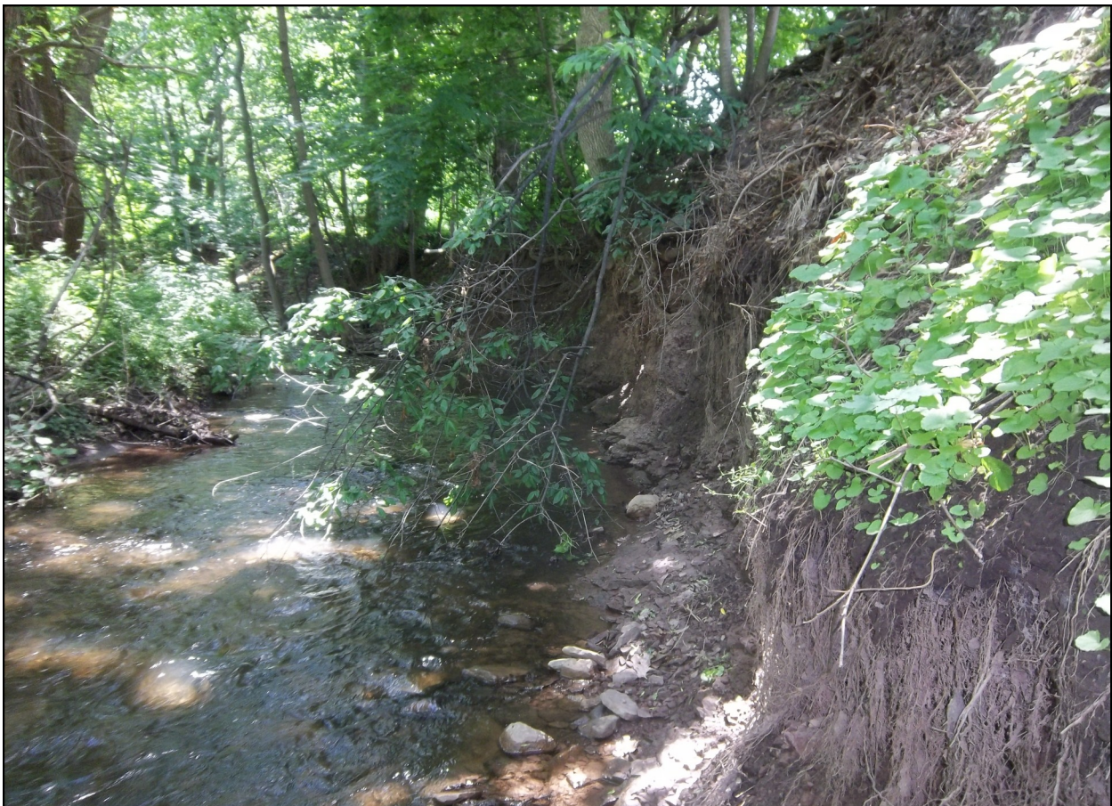
Figure 5. Eroded Streambank (just south of Latta Road crossing)
